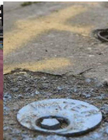
Valves, Vaults and Substructures
